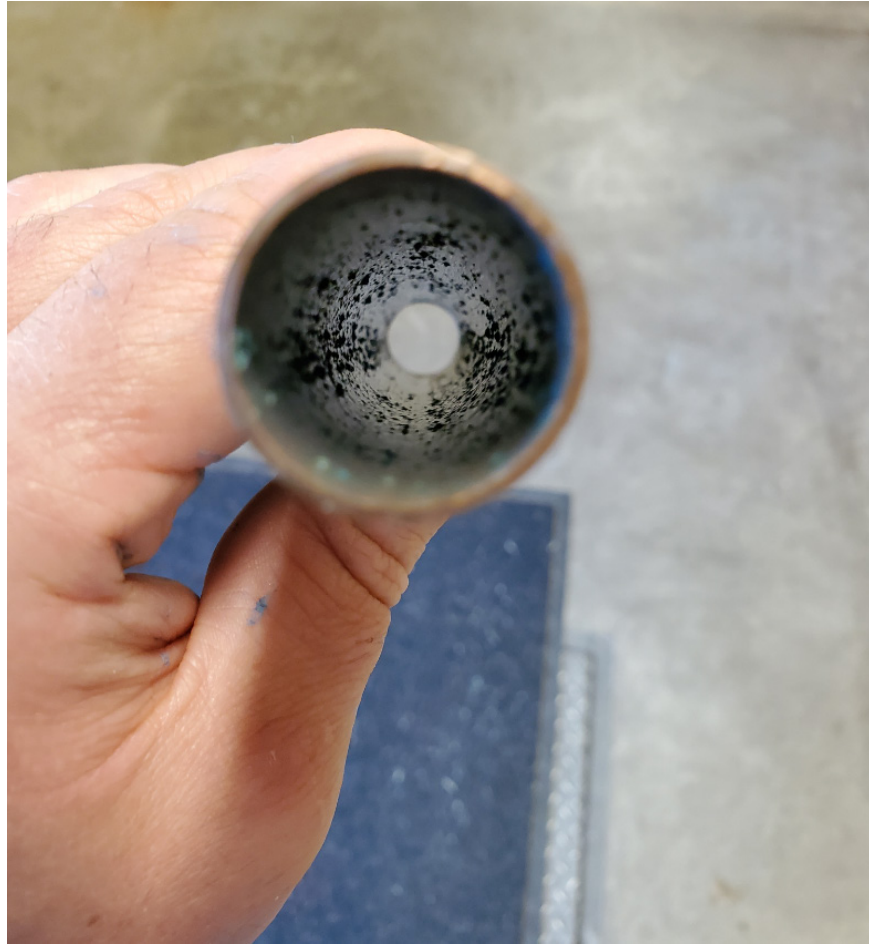
Figure 23 Harvested Pipe Segment Interior Scaling
