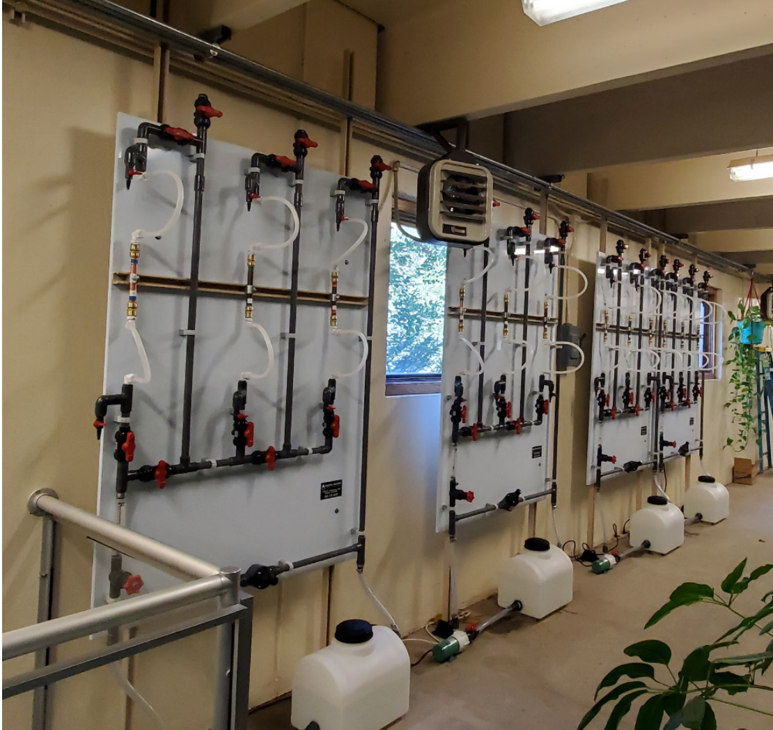
Figure 24 Pipe Loop Panel Area
